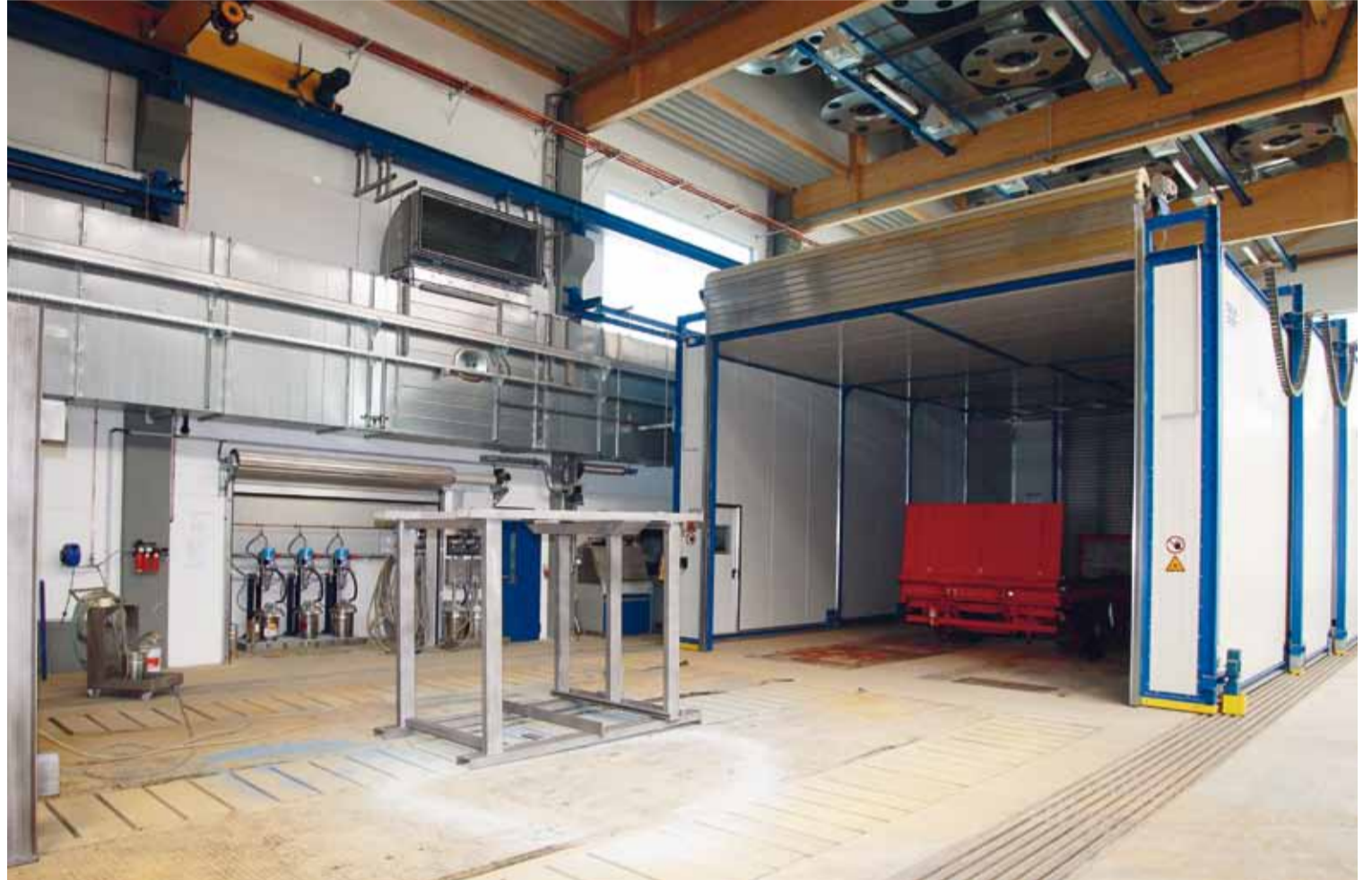
Open-space paint spraying area with movable telescopic dryer.
