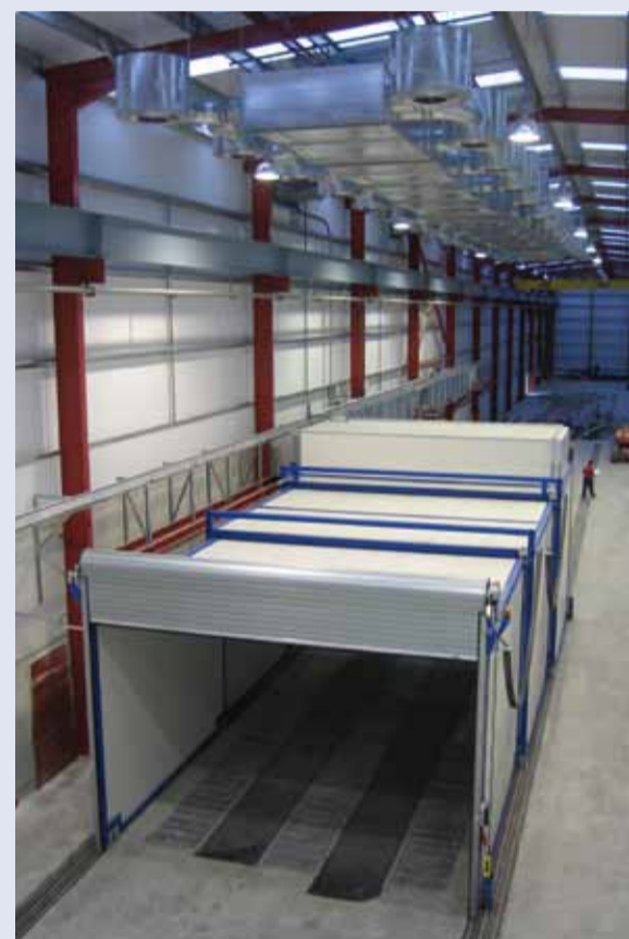
Telescopic dryer on an open-space paint spraying area.
