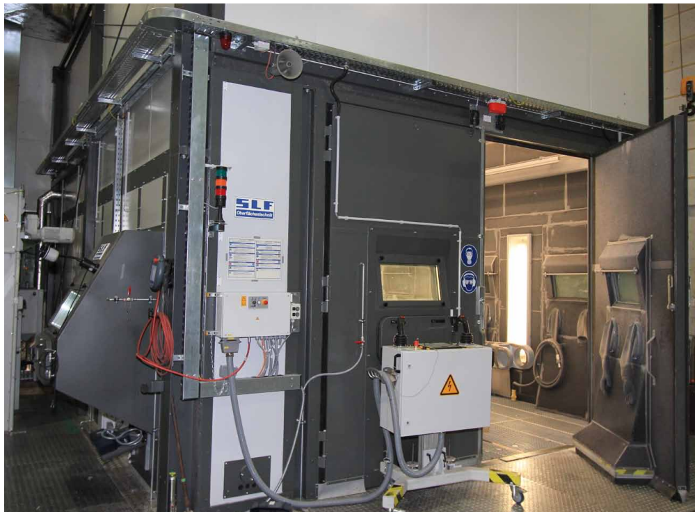
Exterior view of a blastroom with ReCo-Blaster®
